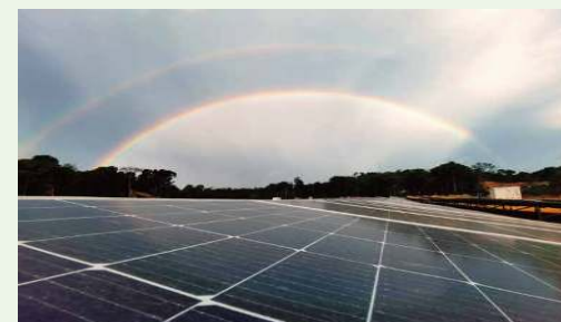
Photovoltaic Panels at Aurora Gold Mine
