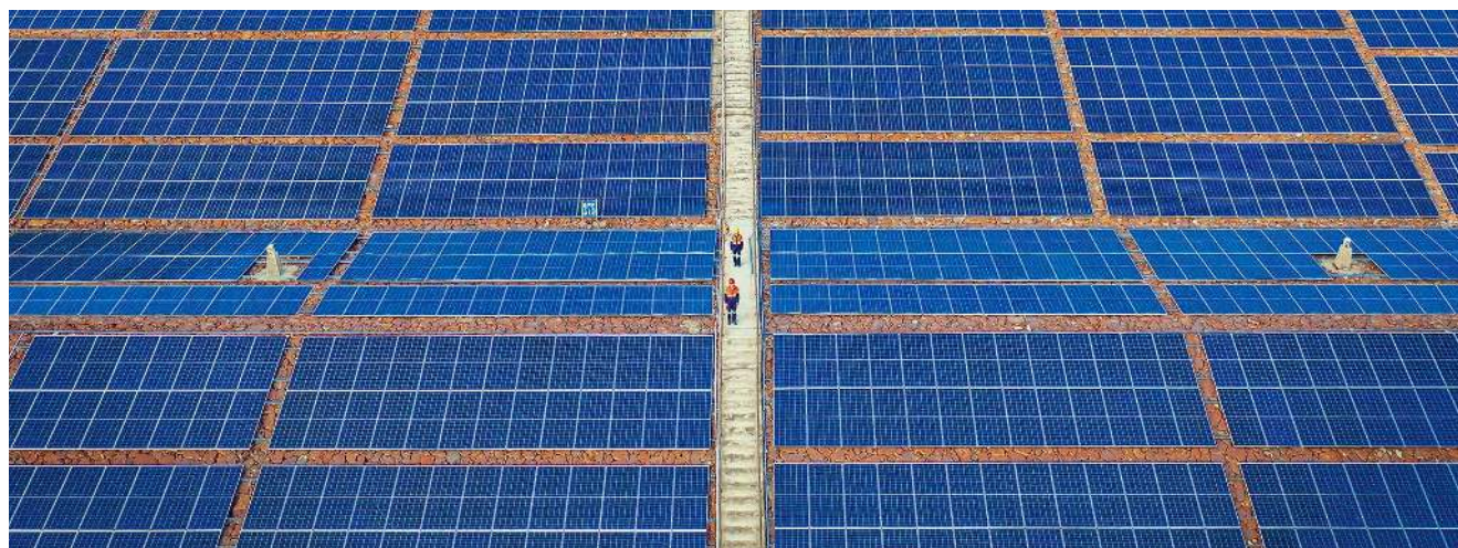
Photovoltaic Panels at Zijinshan Gold-Copper Mine
