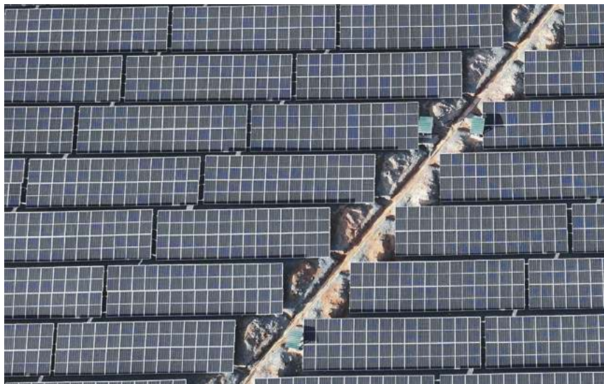
AGM's solar power array
