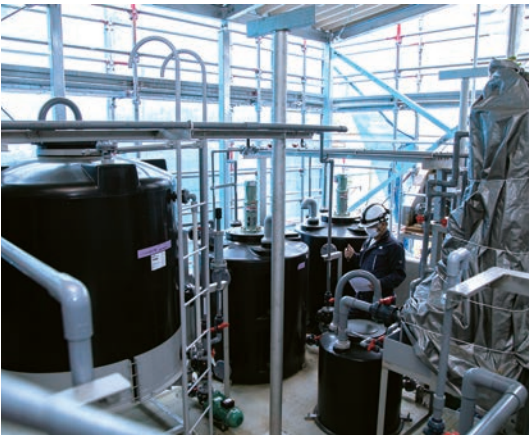
Installed equipment (as of May 2023)
