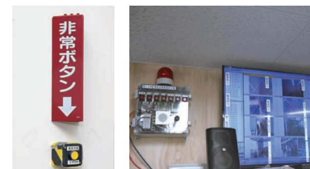
Emergency support switches and monitors
