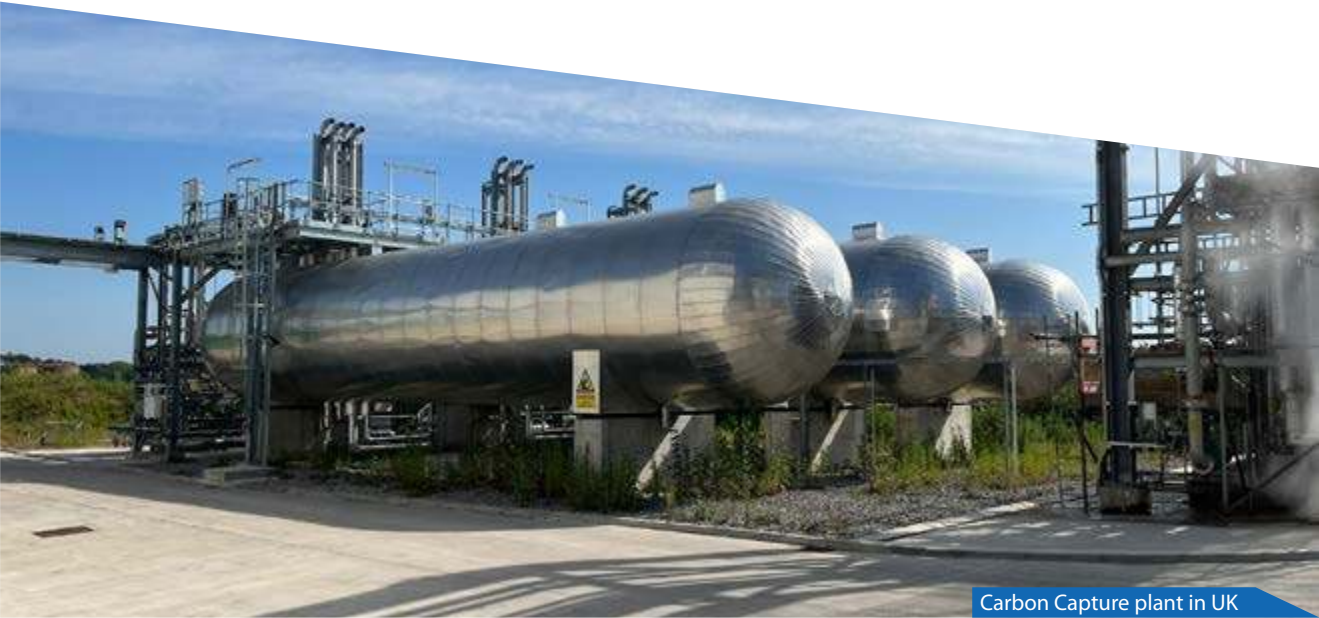
Carbon Capture plant in UK
