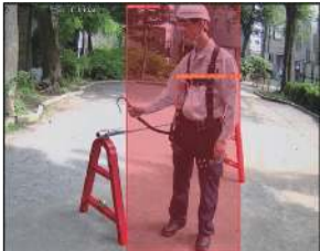
Unsafe (hook disengaged)
