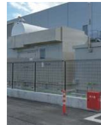
On-site power generation at Miyagi Distribution Center
