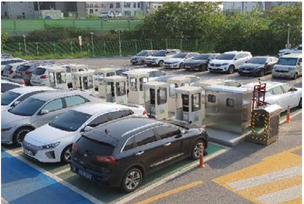
EV charging area at our Giheung worksite
