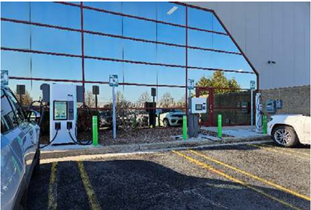
EV charging area at our America corporation(SDIA)
