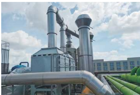
Sunny Zhejiang Optics Exhaust Gas Treatment Facilities
