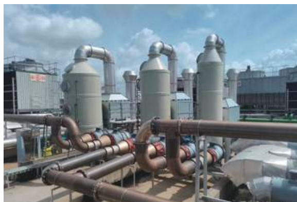
Sunny Zhejiang Optics Exhaust Gas Treatment Facilities
