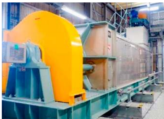
Dehydrator installed at Naoetsu Plant
