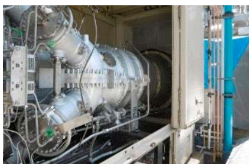
Gas turbine generator
