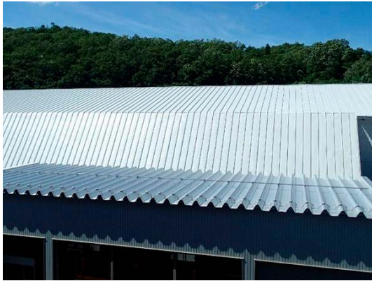
Roof with heat-shielding paint
