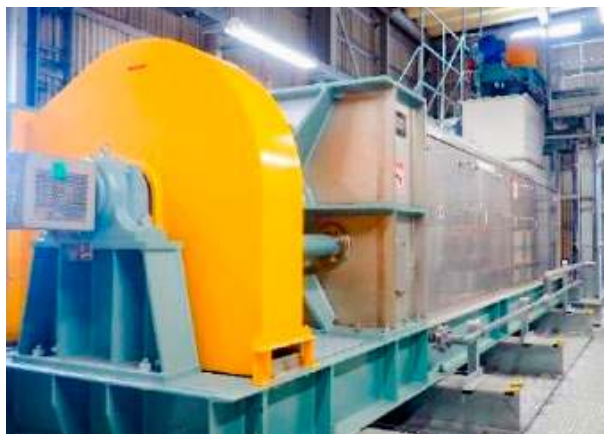
Dehydrator installed at Naoetsu Plant
