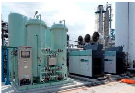
Nitrogen recovery equipment
