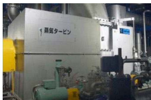
Steam turbine generator
