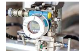
Water and gas meters
