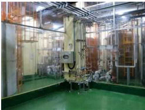
waste liquid tank.jpg
