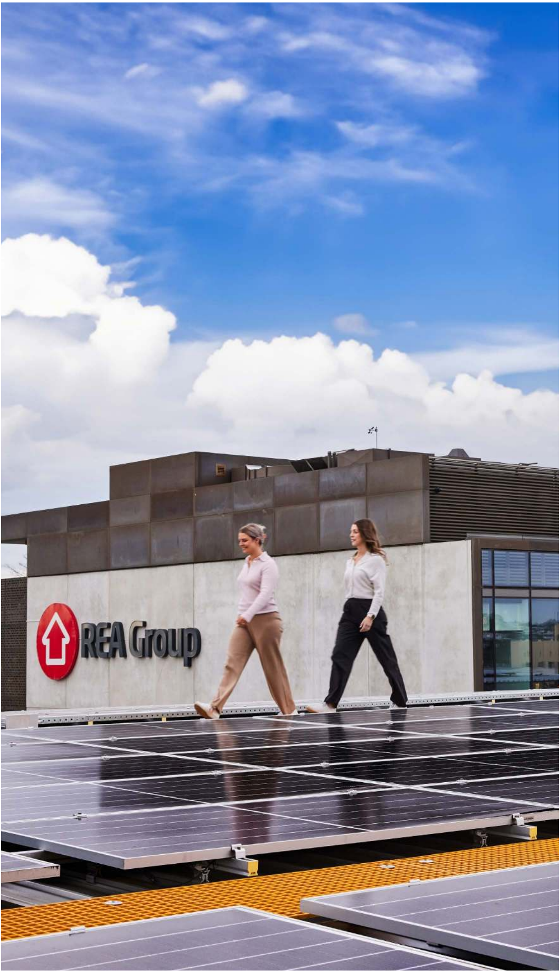
Solar panels at REA Group’s head office in Melbourne
