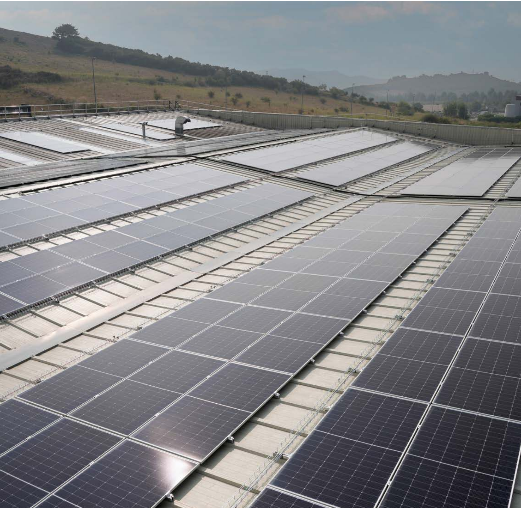
Solar panels installed on the Calle Alto de Armentia supermarket in Vitoria-Gasteiz, Araba/Álava.
