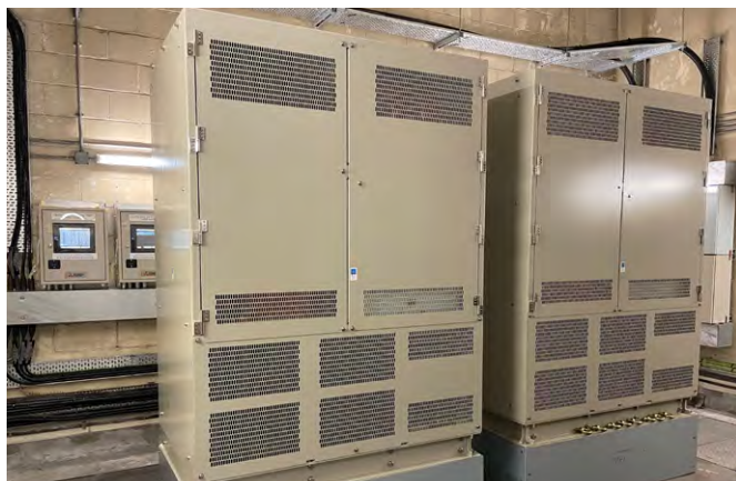
Energy Saving Inverter systems at station
