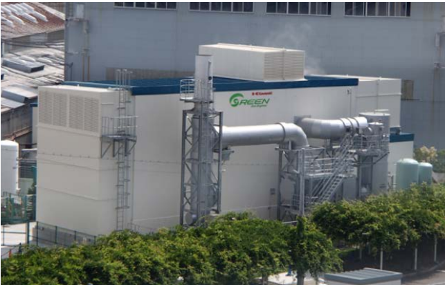
Gas cogeneration system to be introduced (Photograph: Kawasaki Heavy Industries, Ltd., Kobe Plant Power Center No. 3)
