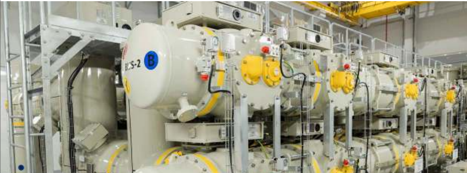
132 kV ESKAN YALAYIS Substation, UAE
