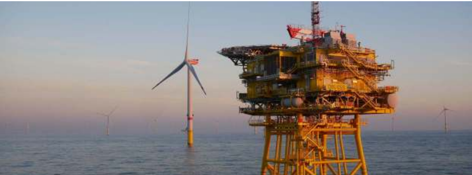
HVAC Offshore Substation
