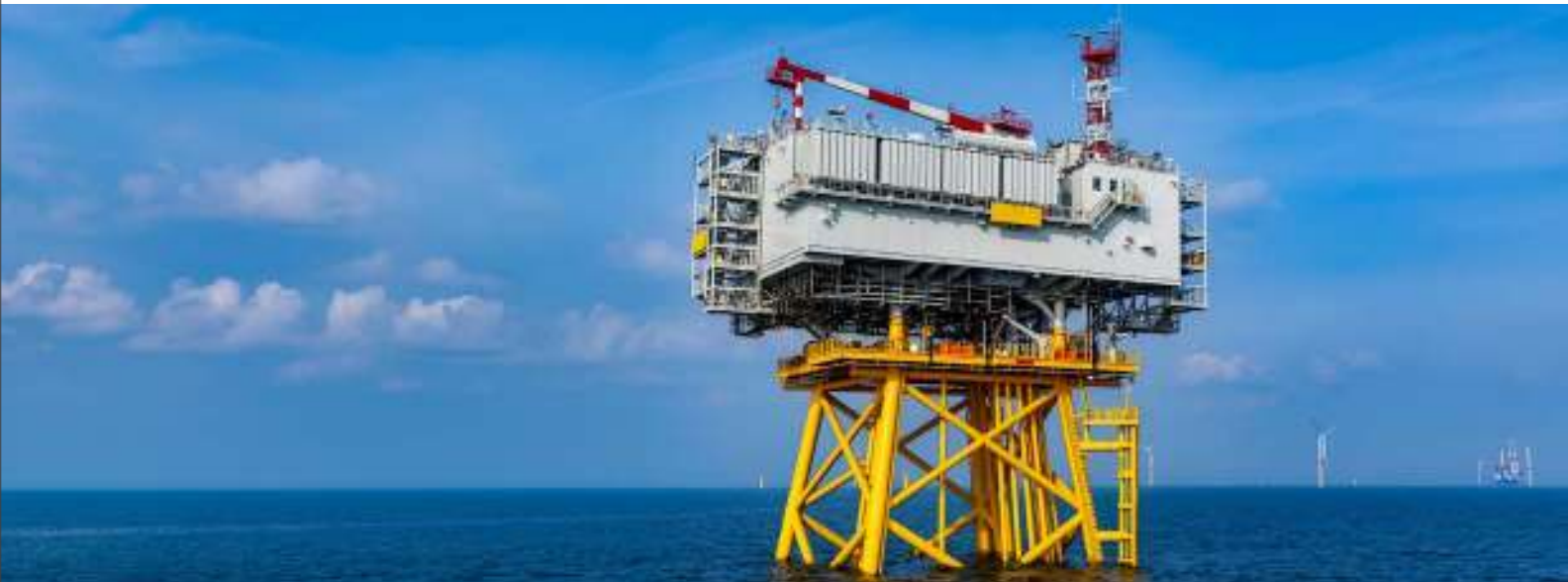
HVDC Offshore Substation
