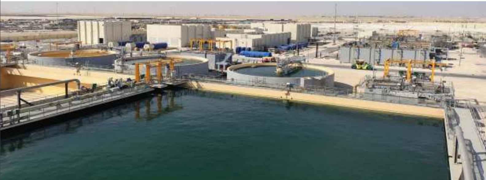
10 MLD Integrated Industrial Effluent Treatment Plant, Qatar
