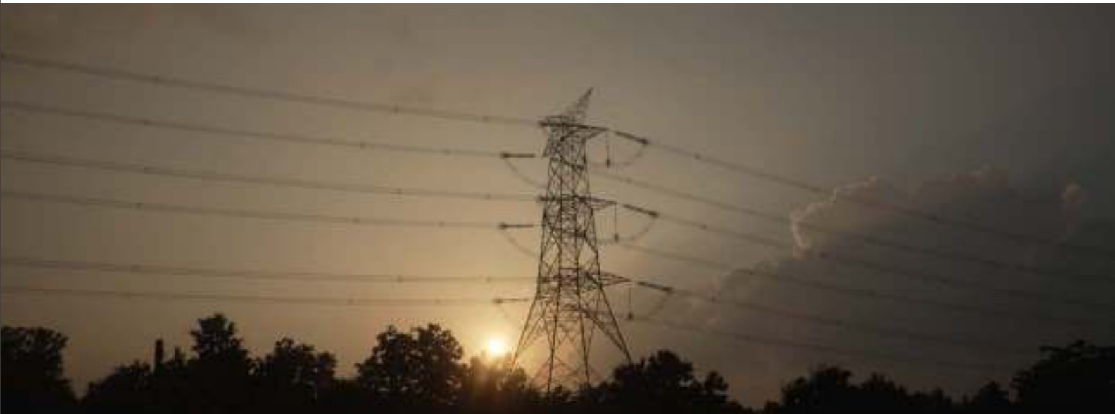
765 kV Navsari–Phadge Transmission Line, Gujarat
