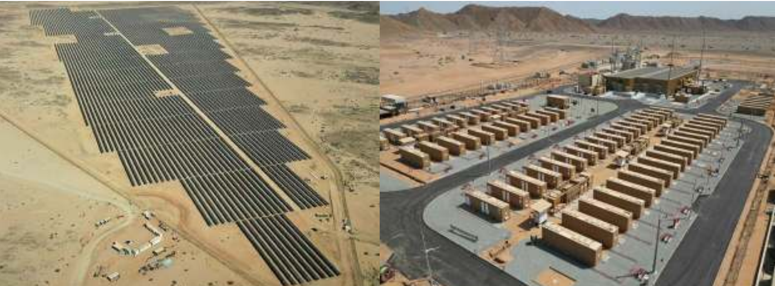
AMAALA Utilities PPP Project in Kingdom of Saudi Arabia, featuring a 250 MWp solar PV plant combined with over 750 MWhr of battery energy storage
