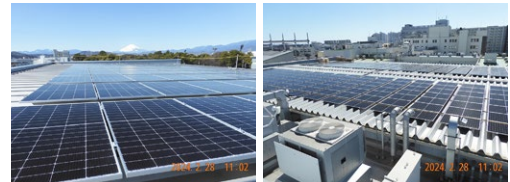
Installed solar panels
