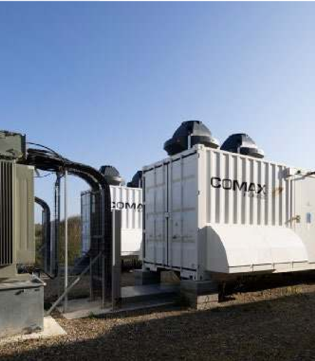
Comax France’s battery energy storage system in Pacy-Sur-Eure (France).
