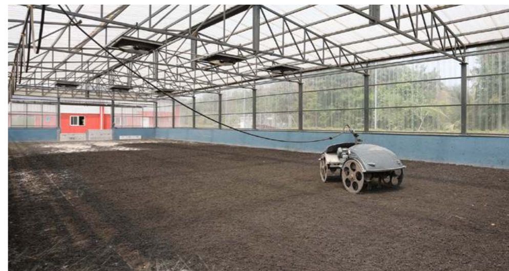
Solar sludge drier in Infosys Hyderabad
