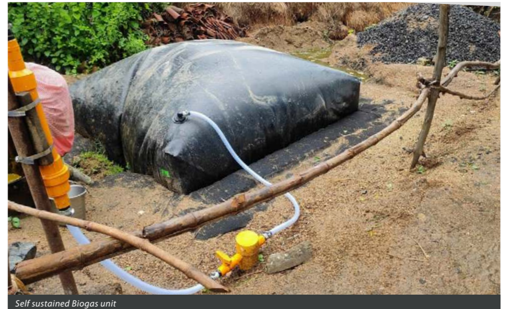
Self sustained Biogas unit
