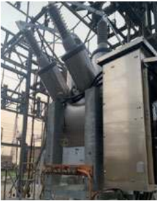
A circuit breaker is pictured at Manby TS
