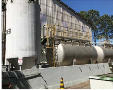
Rainwater storage facility (FUJIFILM do Brasil Ltda.)
