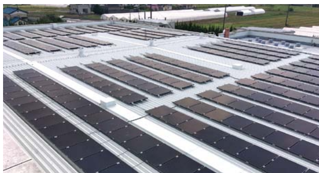
Photovoltaic power facility in FFTP Sano Site
