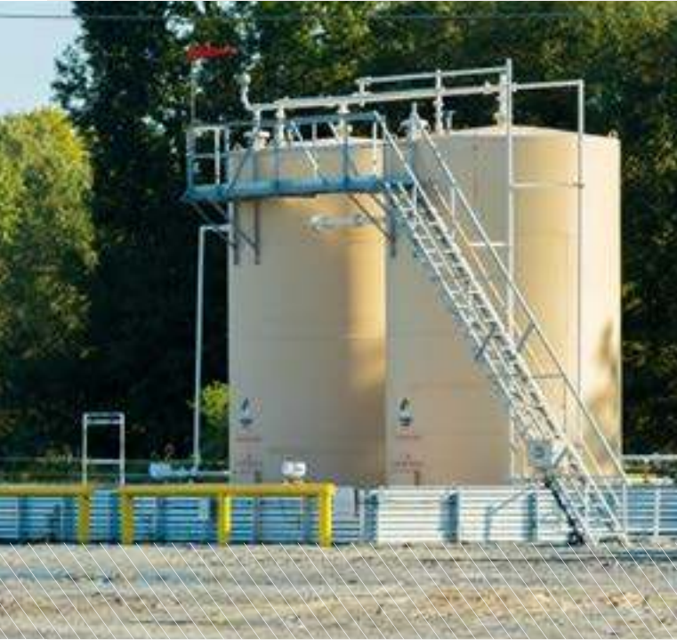
Each production site features secondary containment, such as a berm, to prevent spills from reaching the surrounding environment.
