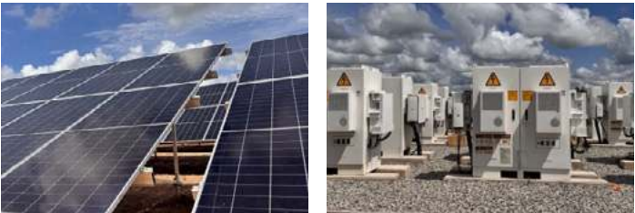
A 500kW solar PV plant with battery storage, the first of its kind, now powering over 1 933 Limpopo connections.
