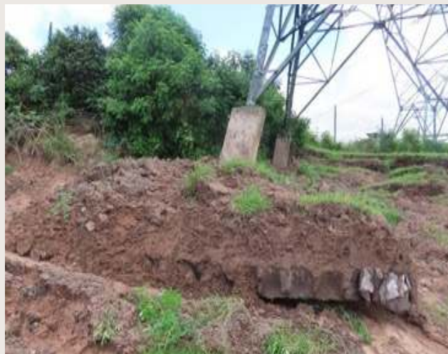
Mudslide and tower damage
