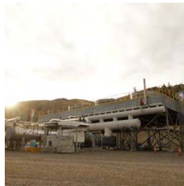
Page 41 Compressor station located near Savona, BC, along our natural gas transmission pipeline.
