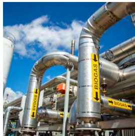
Page 29 The StormFisher RNG facility located near London, ON, uses upgrading equipment to turn food waste into pipeline-quality gas, which is then injected into the Enbridge Gas network in Ontario.
