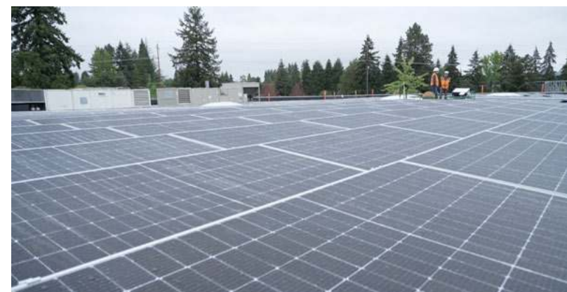
Dynaelectric Oregon completed this new solar installation for a manufacturing facility, helping the client achieve their sustainability goals and minimize operating costs.
