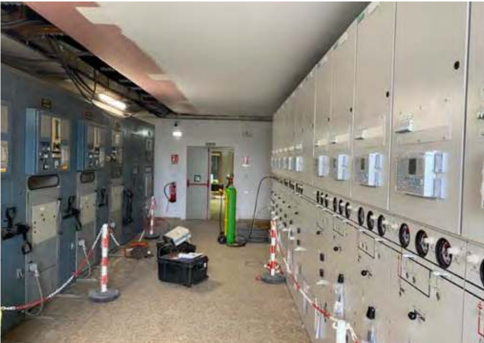
New bays in the Langreo substation
