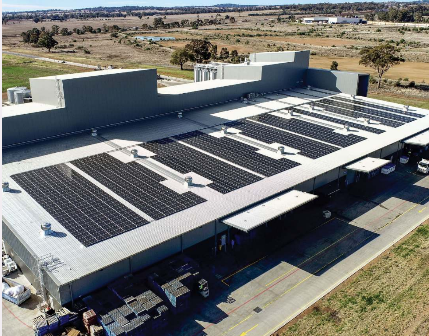
Roof-mounted solar array at Parkes, NSW
