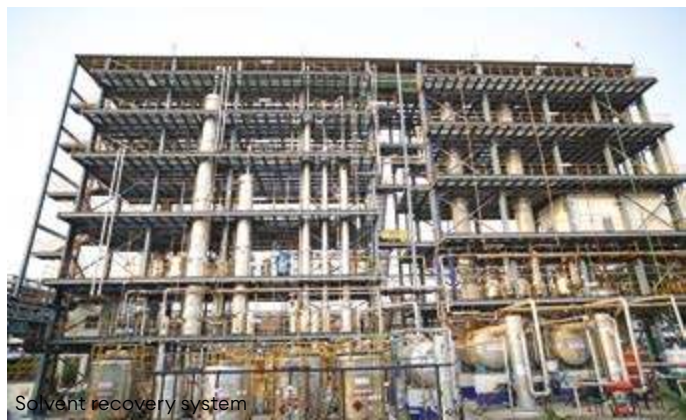
Solvent recovery system
