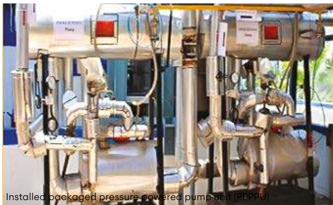
Installed packaged pressure powered pump unit (P3PU)
