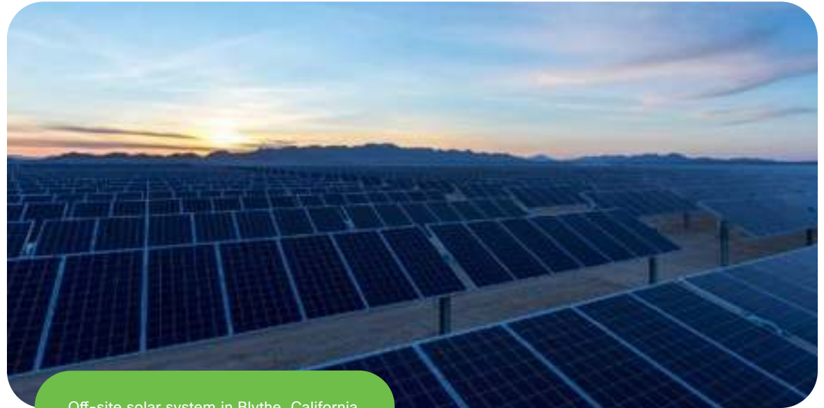
Off-site solar system in Blythe, California
