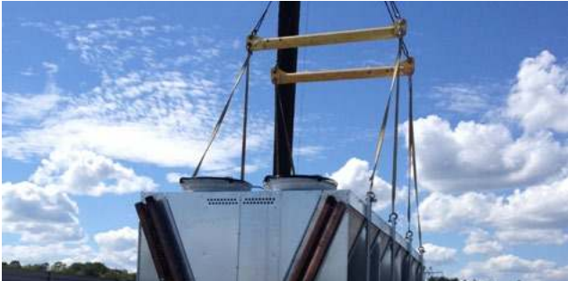
Dry Cooler Unit Saves $280,000 per Year, Ontario, Canada
