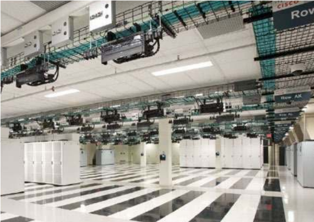
Cisco Data Center, Research Triangle Park, North Carolina
