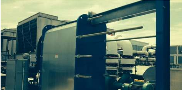
Heat Exchanger Saves over $400,000 per Year in Energy Costs, San Jose, California
