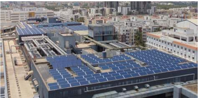
Solar Project at Cisco Office Building, Bangalore India
