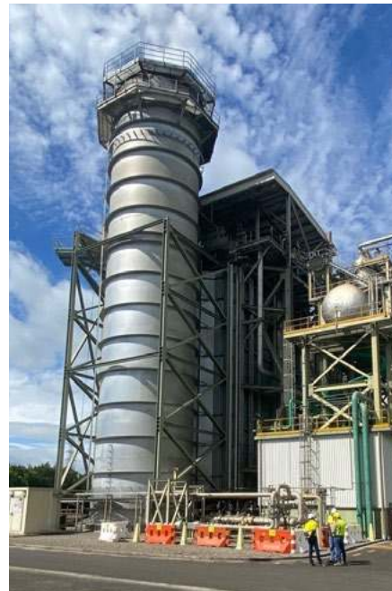
TCC's Heat Recovery Steam Generator at Stratford.
