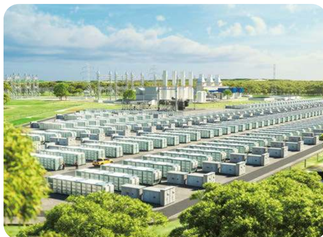
■ EnergyAustralia invests in flexible capacity initiatives such as the Wooreen battery energy storage system in Victoria to support Australia's clean energy transition.
