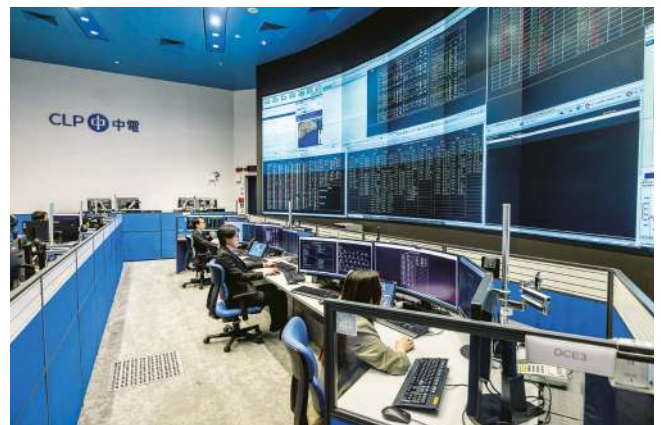
CLP Power's System Control Centre, which marked its 40 th anniversary in 2025, has been operating round the clock to monitor the power system, ensuring a stable and secure electricity supply.
