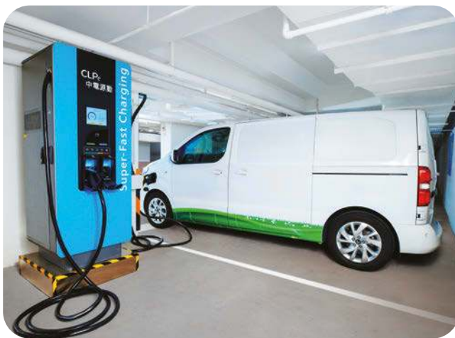
■ CLPe's new network of EV charging stations in Hong Kong helps meet growing charging demand from commercial vehicle fleets.
