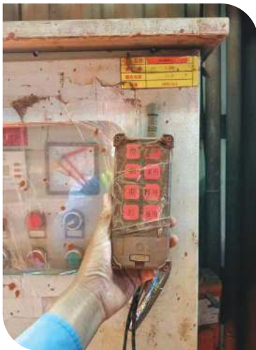
Interlocking Device Controllers
