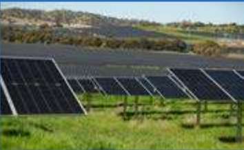
Front cover: Lightsource bp solar farm, Wellington North NSW
