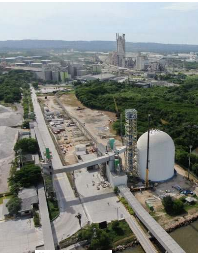
Silodome in Cartagena plant
