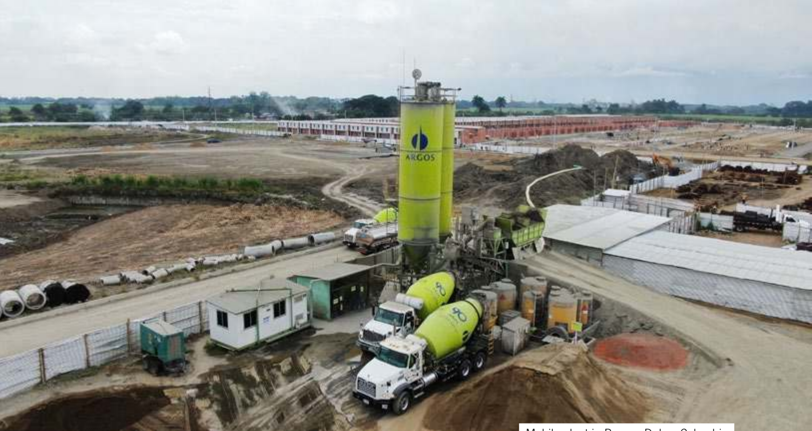
Mobile plant in Parque Dulce, Colombia
