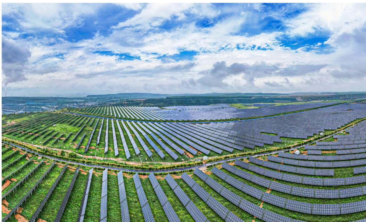
Pingshuo Group 100MW photovoltaic project
