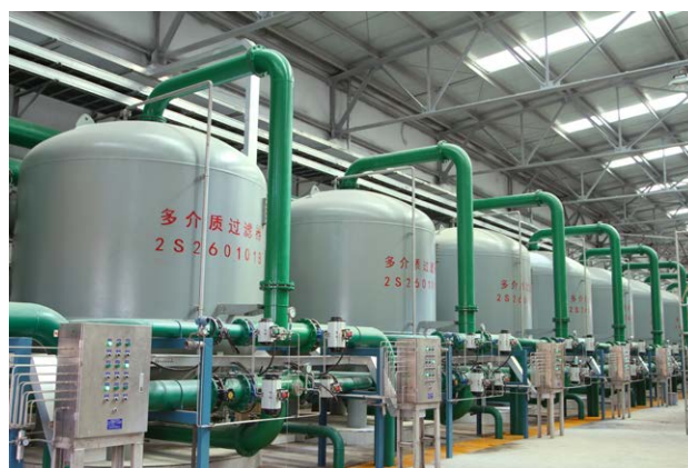
Treatment Device of Ordos Energy & Chemical Company
