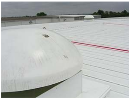
Electric rooftop exhaust fans for heat discharge
