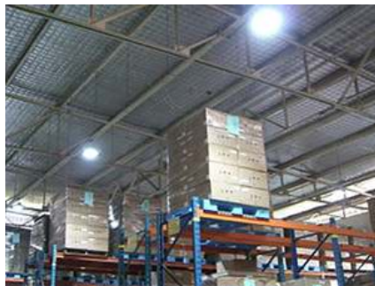
Daytime warehouse lighting
