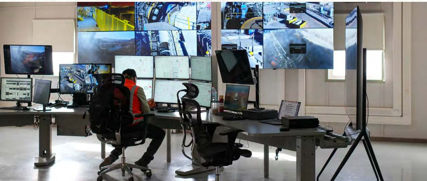
Mantoverde – Concentrate Plant Control Room
