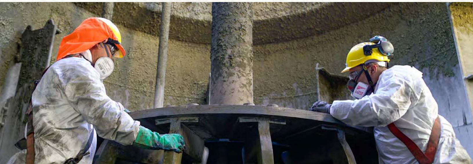
Mantoverde – Plant Maintenance
