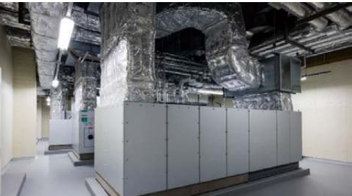
High-efficiency air conditioners upgraded for clean rooms
