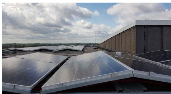
Solar panels at Canon Production Printing Netherlands
