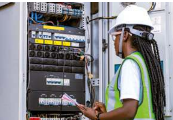
Energy Systems Maintenance - Cameroon
