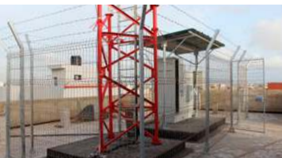
Energy equipment on an ESCO site - Senegal
