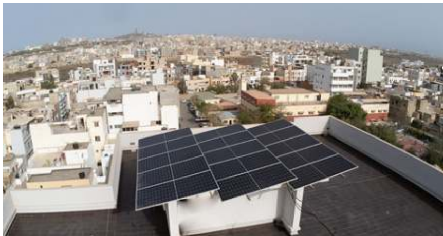
Solar panels on a technical building - Senegal
