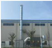
Fume Treatment Equipment
