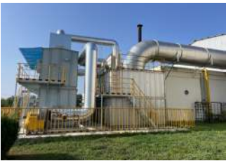
RTO Waste Gas Treatment Equipment
