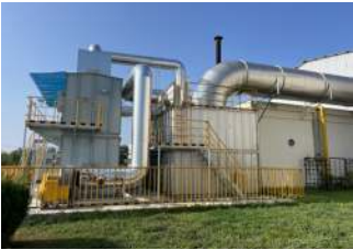
RTO Waste Gas Treatment Equipment
