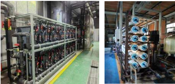
Demineralized Water Preparation System
