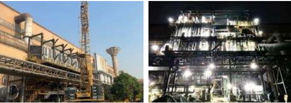
Enhanced waste heat recovery boiler
