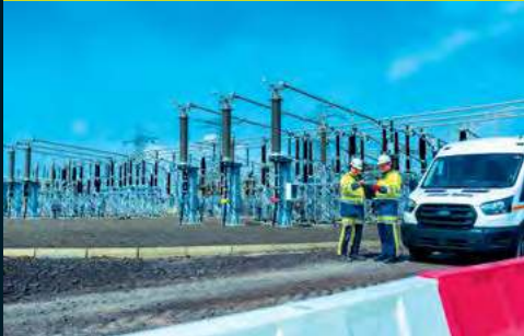
Tealing Substation, Scotland for SSEN Transmission.
