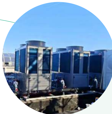
▲ Application of air source heat pump technology
