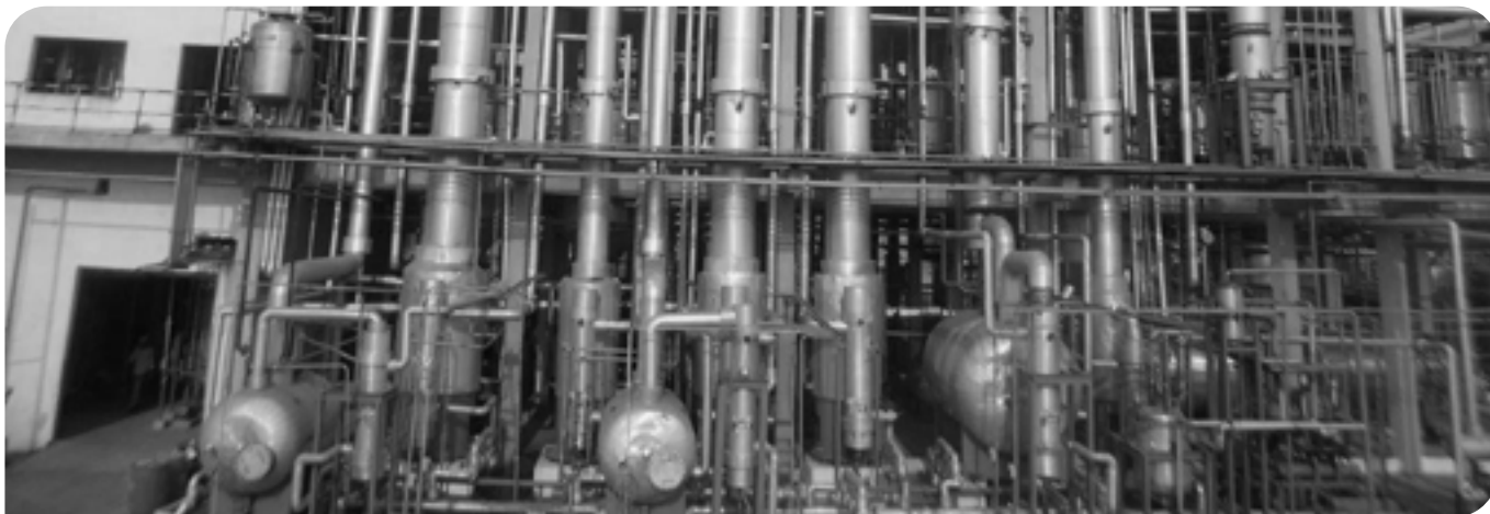
Solvent Recovery plant
